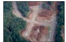
Paving the way to a new suburban subdivision in what was once forest land.
